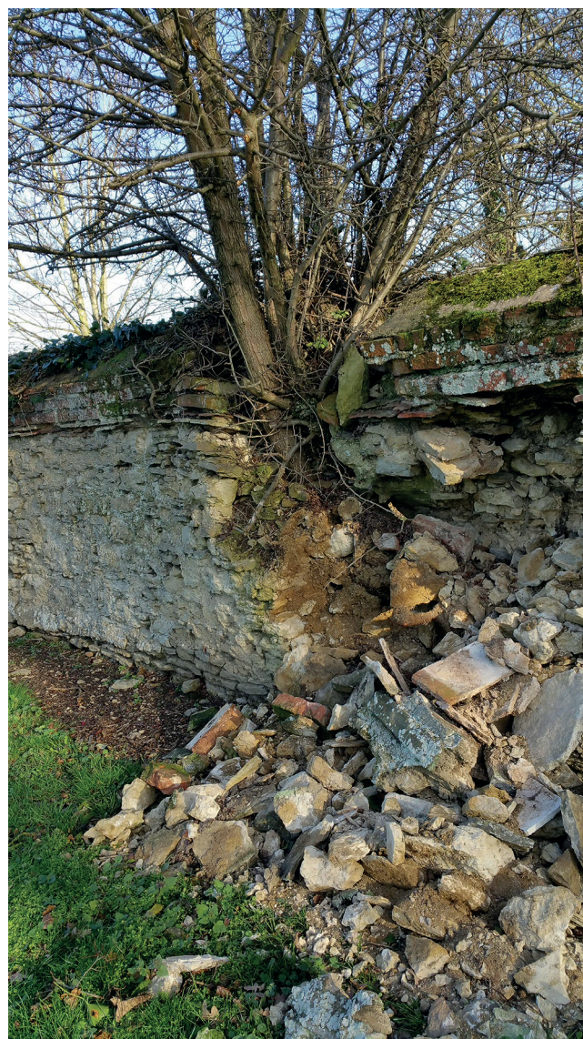
Figure 6: Damage to the northern wall caused by Storm Doris
